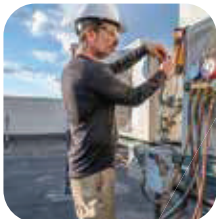
Heat, Ventilation, & Air Conditioning (HVAC)
